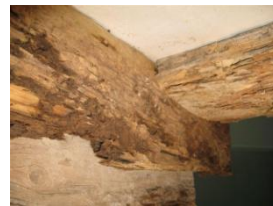
Fig. 2 & 3 Termite attack. Wooden beam destruction by Termites
